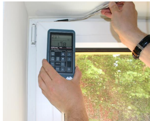
Measurement of the air speed during the pressure test at a window not yet correctly adjusted, using an anemometer
